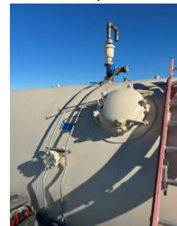
Air Scour System Mods
