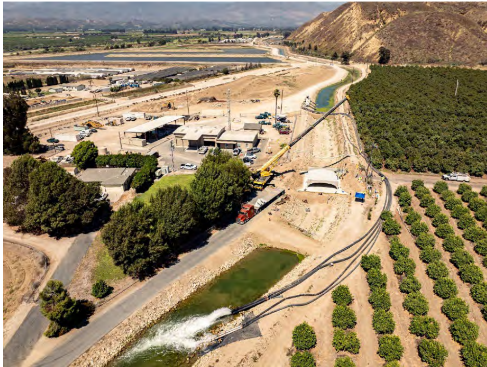
Figure 6 - Inverted Siphon Replacement Project precast bridge was set by crane in 10 pieces on August 14. The pumping bypass is also shown.
