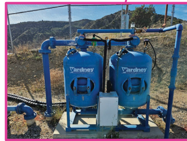
LP WTP Pre-Filters to Be Replaced
