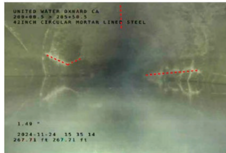
Hinge Cracks Approx. STA 223+64.38
