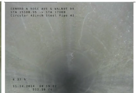
Multiple Cracks Approx. STA 164+26.55
