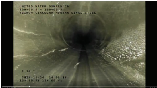
Lining Pitting Approx. STA 219+62.38
