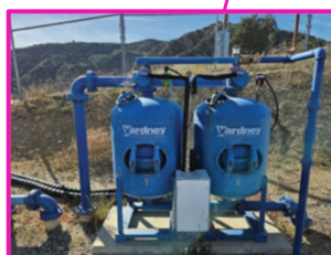
LP WTP Pre-Filters to Be Replaced
