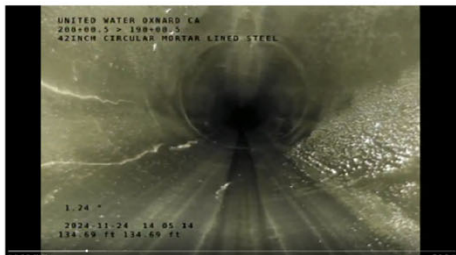
Lining Pitting Approx. STA 219+62.38
