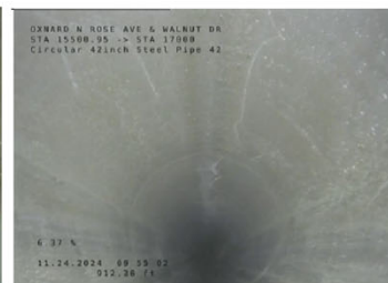
Multiple Cracks Approx. STA 164+26.55
