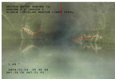
Hinge Cracks Approx. STA 223+64.38
